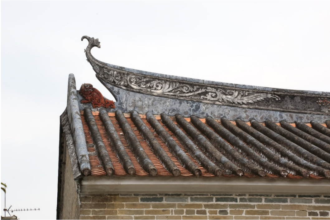
The plaster sculptures with lion and grass motif ornamenting the main ridge of the rear hall
