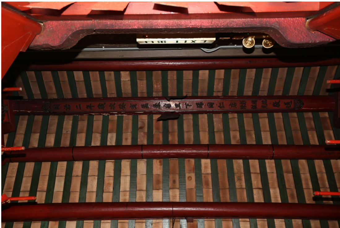
Inscriptions on the ridge purlin of the entrance hall marking the 2 nd year of the Tongzhi (同治) reign (1863) of the Qing dynasty
